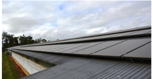
Figure 7: Some of the panels that make up Will's 90kW solar PV system
