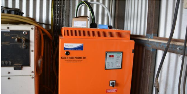
Figure 2: Power factor correction (PFC) device installed in 2013
