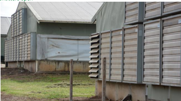
Figure 6: Some of Will's sheds lack discharge cones and actuators to hold shutters open
