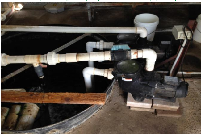
Figure 2: Pumping systems like this one make up the bulk of the energy use on site. Finding a more efficient pump could save about $3,000 a year.
