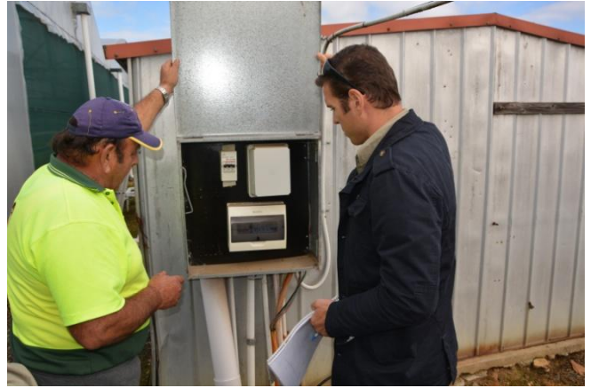
Figure 3: Farmer Joe D’Anastasi and Leigh Rostron from Energetics examine electrical equipment outside one of the pump sheds on site.
